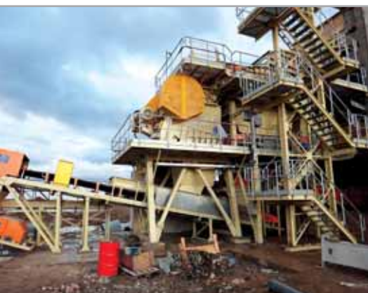
Jaw crusher DCJ 1400x1120 – limestone crushing
