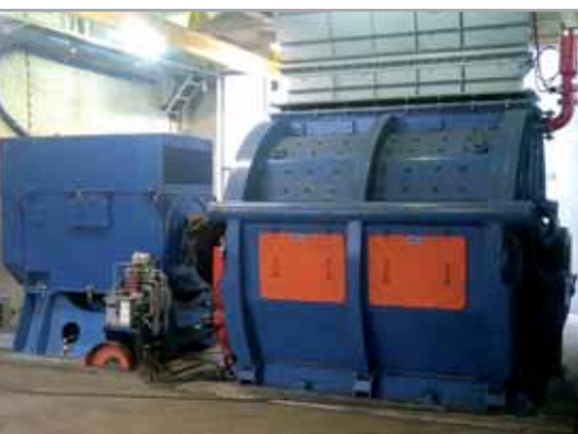
Crusher KMR 1824 – coal crushing 350t/h
