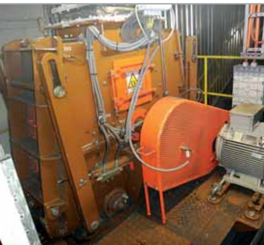
Crusher KMR 0804 – coal crushing 8t/h
