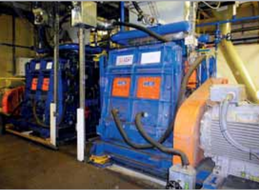
Crushers KMR 0808 – coal crushing 2x26t/h
