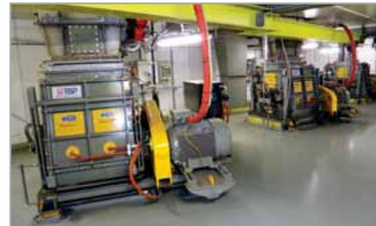
Crushers KMR 0808 – coal crushing 3x14t/h
