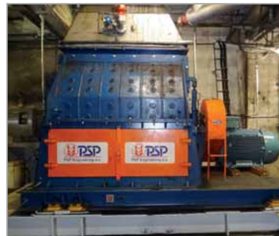
Crusher KMR 1220 – coal crushing 250t/h
