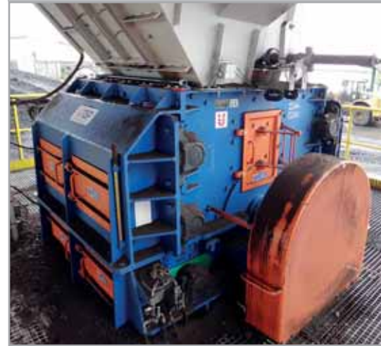
Crusher KDV 1013 – coal crushing 350t/h
