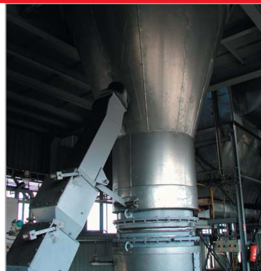
Air separator LTR-R 1650 at the coke grinding plant with 12.5t/h capacity – OKD Ostrava, Czech Republic
