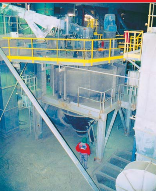
Air separator VTP 2400 at the cement grinding plant with 100t/h capacity – Kujawy, Poland
