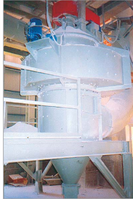
Air separator VTP 1100 at the limestone grinding plant for 9 t/h at Redipuglia, Italy
