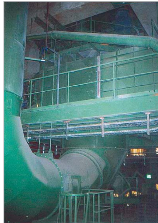
Lower part of the air separator VTP 2900 with exhaust duct at the cement grinding plant for 130 t/h at Anhovo, Slovenia
