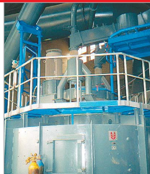
Air separator VTP 2400 at the cement grinding plant with a capacity of 72 t/h – Lukavac, Bosnia and Herzegovina
