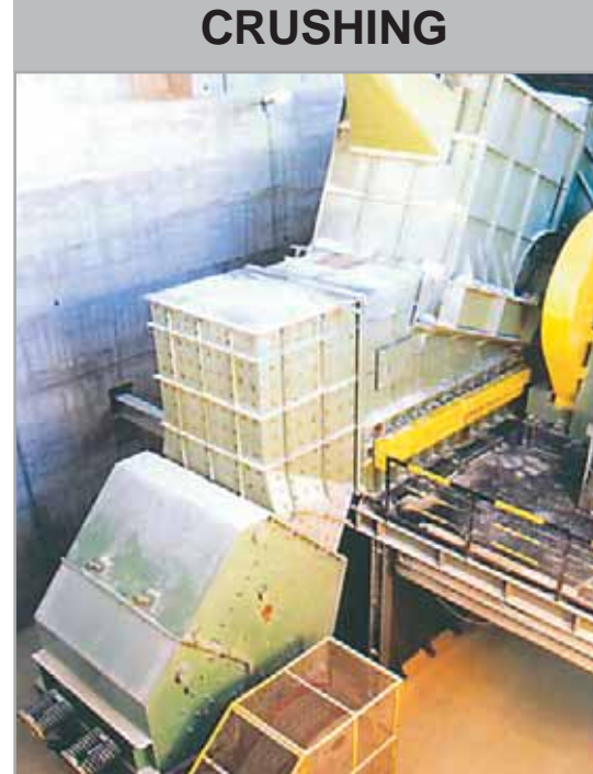
Impact crusher 700t/h – cement material crushing
