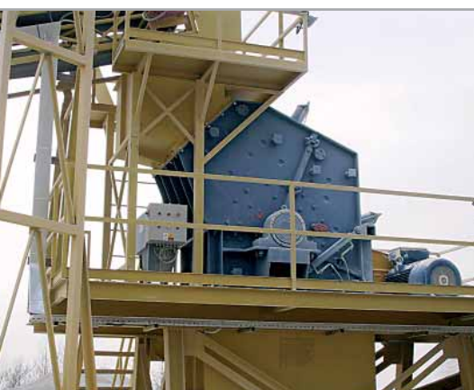
Impact crusher 150t/h – dolomite crushing
