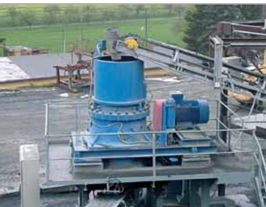
Cone crusher KDC 33 GP – chert crushing
