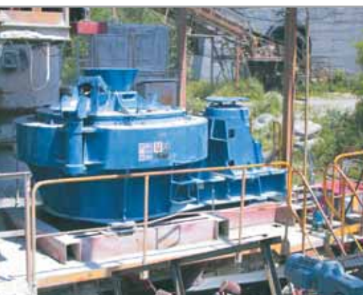
Vertical shaft impactor ODV 1186S – andesite crushing
