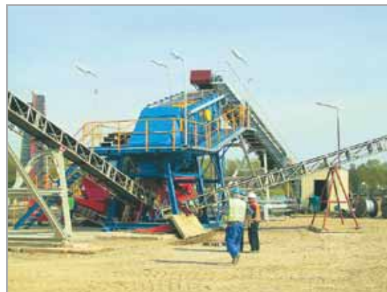
Vibrating screen KDT 1650/3 – gravel sand screening
