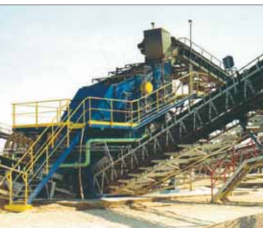
Vibrating screen KDT 2050/3 – gravel sand screening
