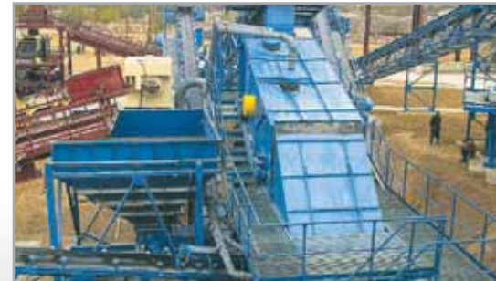
Vibrating screen KDT 2050/2 – granite screening
