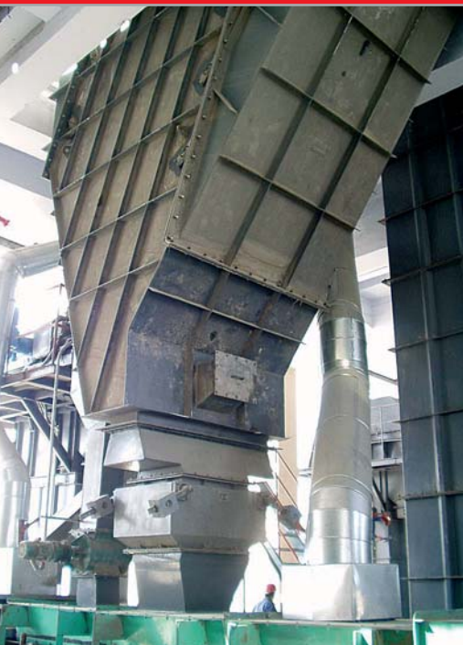
Above: Cascade air separator KVT 1800 as part of the 120 tph cement grinding plant at Qilianhan Cement, China. The photo shows the lower part of the separator with the coarse fraction discharge
